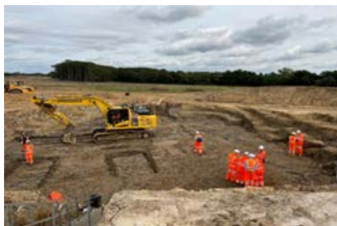
Figure 8 Deep ground investigations were carried out to inform detailed design of the embankments
