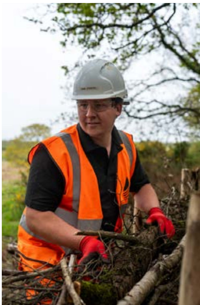
Figure 7 A dead-hedge has been built, creating a barrier to local farmland and a new wildlife habitat
