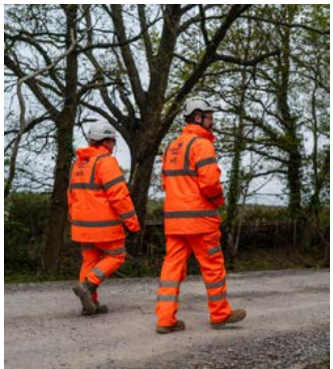
Figure 6 A new northern access road will keep construction traffic away from residential areas
