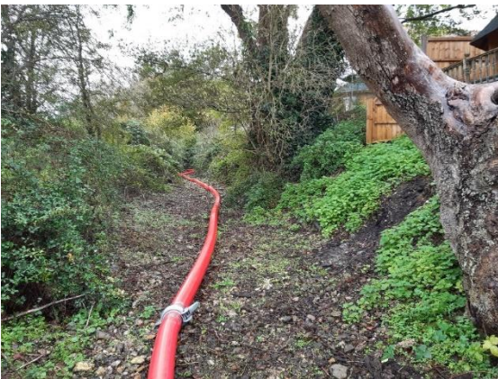
Augmentation pipe in channel (07/11/2022)
