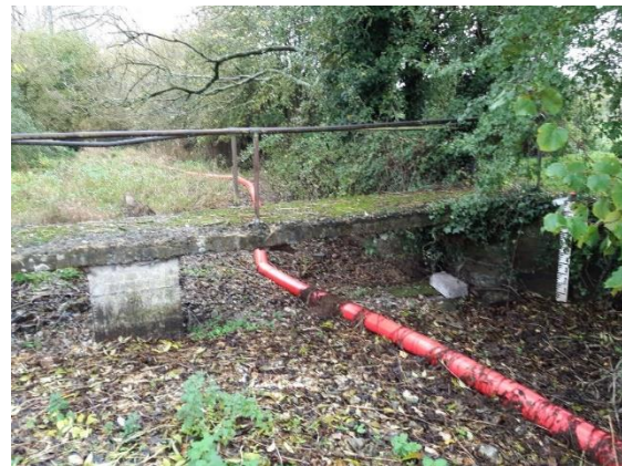
Augmentation pipe in channel (07/11/2022)
