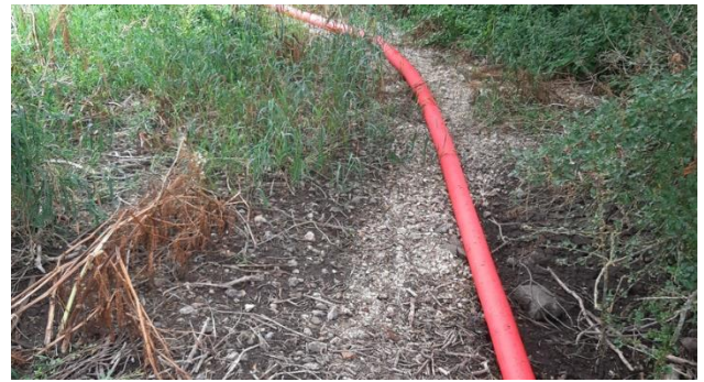
Augmentation pipe in channel at Riverside Cottages (31/08/2022)
