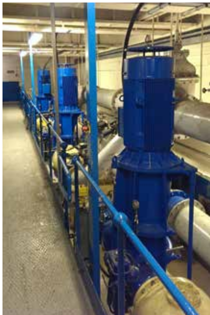
New pumps at Havant Pumping Station
