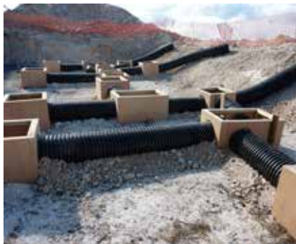
Construction of artificial badger sett at one of the Company's operational sites
