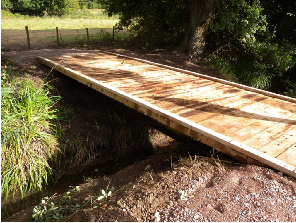
New bridge at the Itchen WTW to enable cattle to access the SSSI flood meadow
