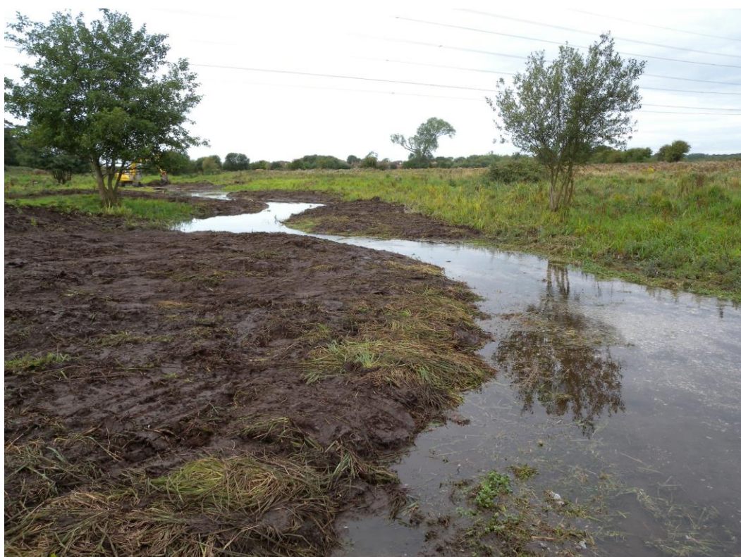
After – River Ems restored channel with meanders, graded edges and gravel base
